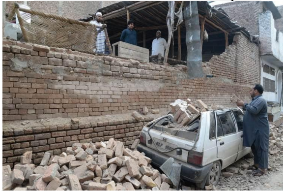
Partial Out of Plane failure of Brick Masonry Wall
